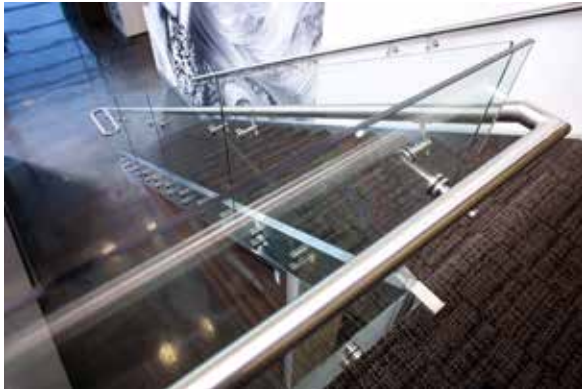
An example of CMPI's glass/stainless handrail systems. They can both fabricate and install this type of work on-site.
