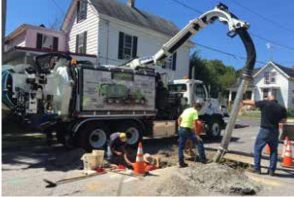
Hi-Vac Aquatech unit on-site demonstration.
