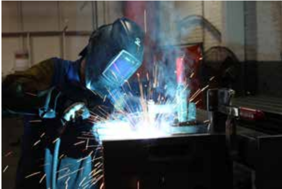
Jensen Metal welders are AWS D1.1-2008 certified, ensuring a quality product every time
